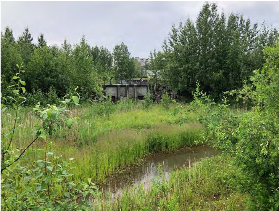
Figure B-20. ANC-04255, Knik Arm Power Plant Concrete Structure, built circa 1950; view to the south
