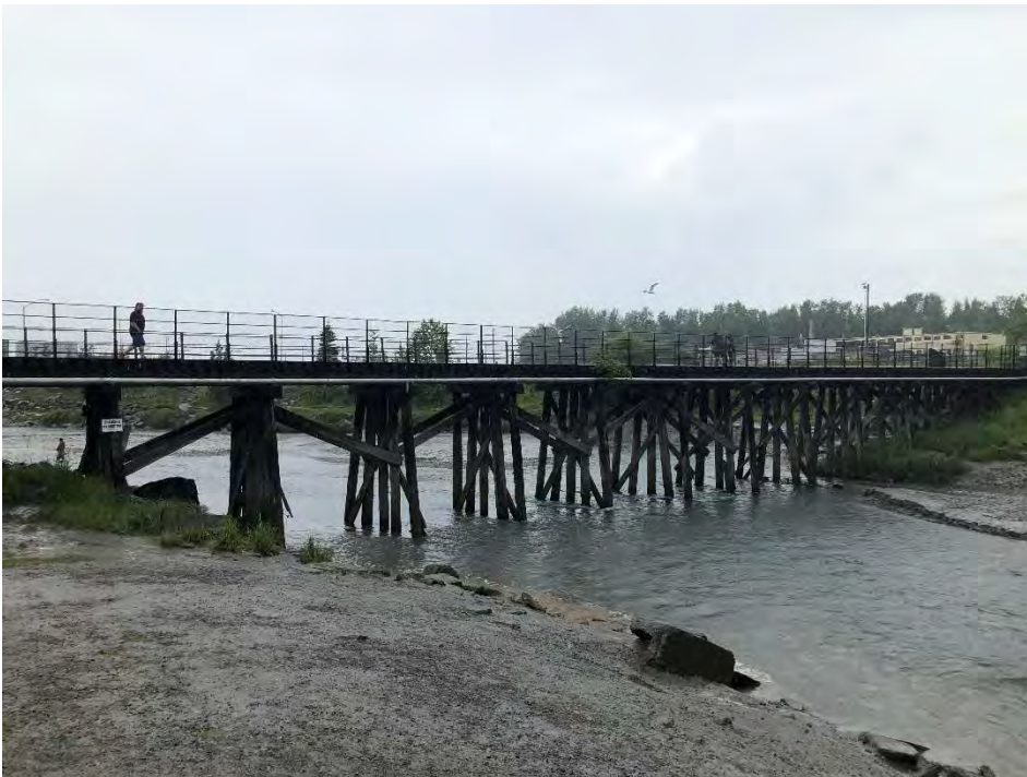
Figure B-11. ANC-02775, Alaska Railroad Timber Bridge at MP 114.6, built in 1956; view to the northwest
